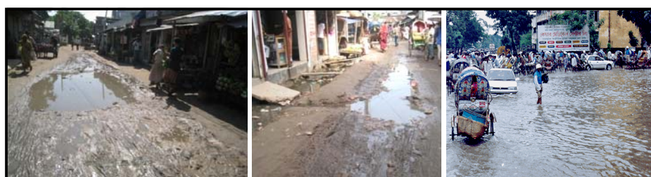
Poor condition of roads in the study area during pre monsoon and flooding period
