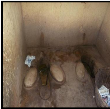
Figure 14: Dirty stained walls, urine on the floors
