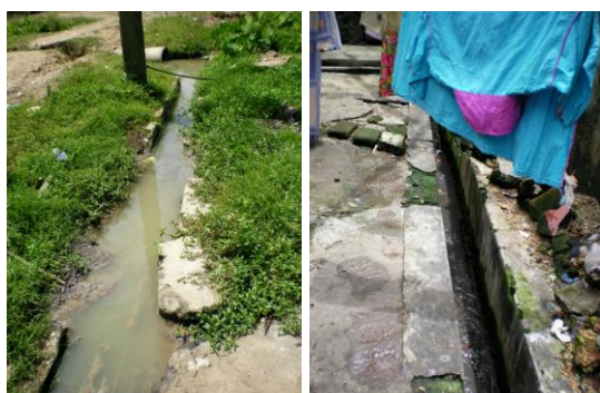
Figure 15: Condition of drainage facilities in original settlements
