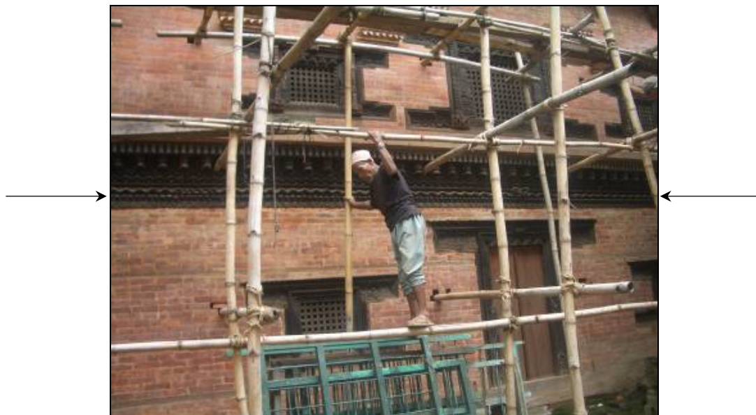
Figure 11: The Naag band around the wall of 55 Windowed Palace in Bhaktapur and the traditional scaffolding made of bamboo ( Referred page 42, footnote:11)
