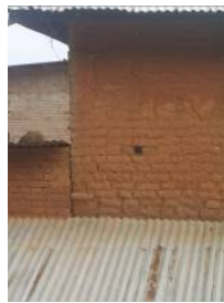
Figure 7: Minor cracks seen on the external wall of the dwelling
