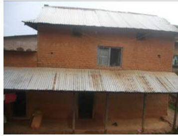
Figure 6: Dwelling which survived 1934 earthquake (referred: page 33, Footnote 5)
