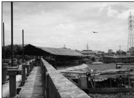
Figure 6.16: The temporary pump station at Rampura with 20 sluice gates Source: Author, 2008
