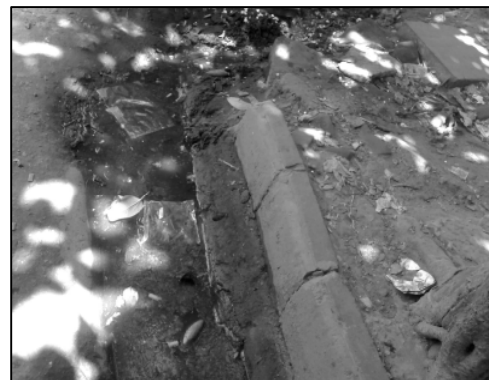
Figure 6.10: The clogged surface drain
