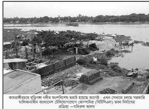
Figure 6.11: The construction work of BTCL building in the Buriganga River Photographer: Monirul Alam
