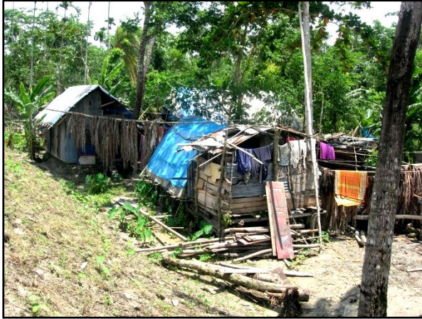
Figure 4.2: Showing house destroyed by Sidr (notice the quality of construction materials), Southkhali Source: Author
