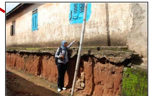
House of Survey Respondent No. 31 with Ms. Mutia Razali pointing to the top of the flood water level height.
