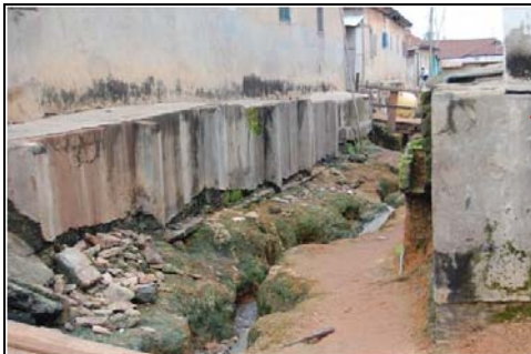
One of the drainage gullies that formed in between the houses in Ayigya Zongo.
