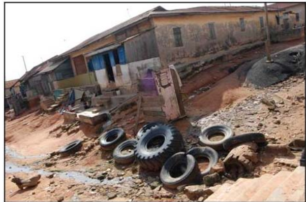
Upper Photo: Portion of the main road in Ayigya with constructed drainage; Lower Photo: Rubber tires used to temporarily hold the soil intact to prevent it from further eroding
