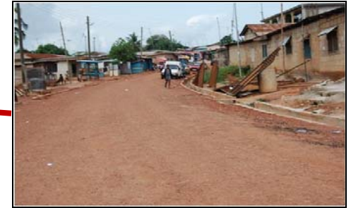
Portion of the main road in Ayigya where concrete drainage has been constructed on what used to be gullies
