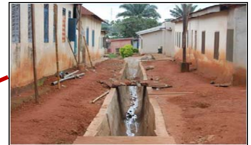
One of the drainage gullies where concrete drainage networks have been constructed in Ayigya Ahimbono
