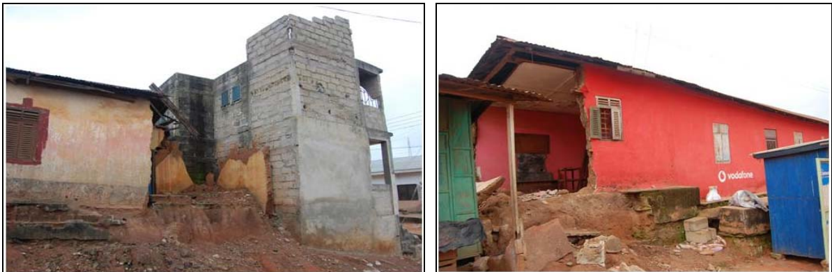
Photos of some houses located in Ayigya Zongo with collapsed portions
