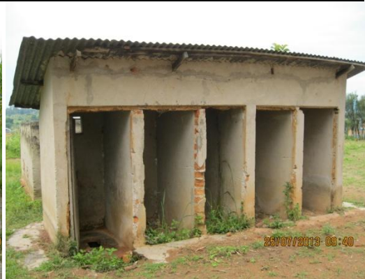
An abandoned latrine at Etori PS due to the removal of all its door shutters. Such incidences were common in all schools.
