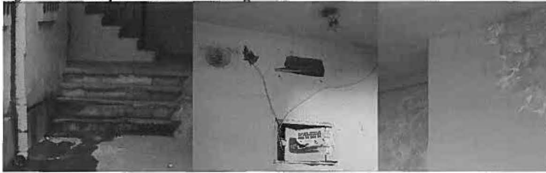
Figure 9: Common problems in older buildings
