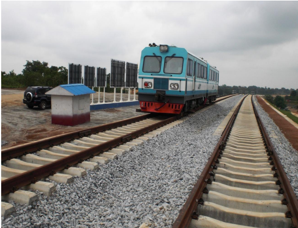
Annex 4: Photograph of the Rail testing train at the rail site used for testing the already laid tracks to confirm standards
