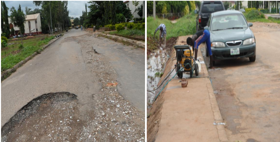
Photograph 4. 2: Road infrastructures, requiring maintenance at Federal Government land, Gwarinpa-Abuja
