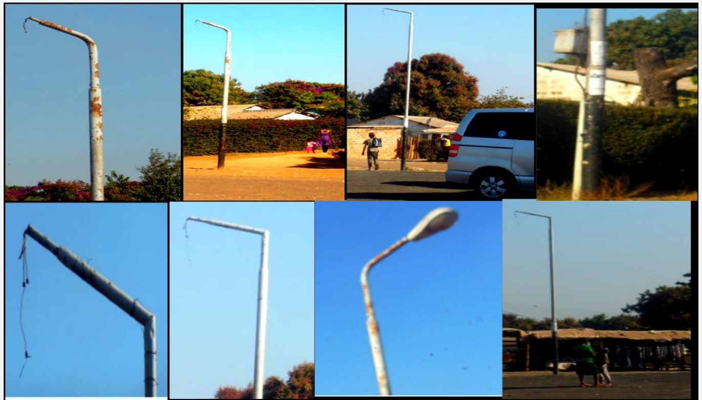
Figure 11: Vandalised Street Lights along Butondo Road
