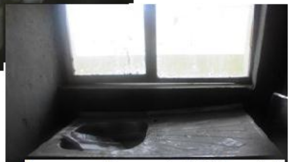
Improper placement of kitchen sink
