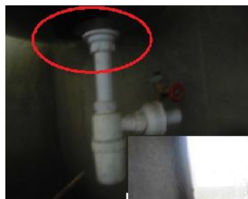
Improper fixing of kitchen-sink fitting
