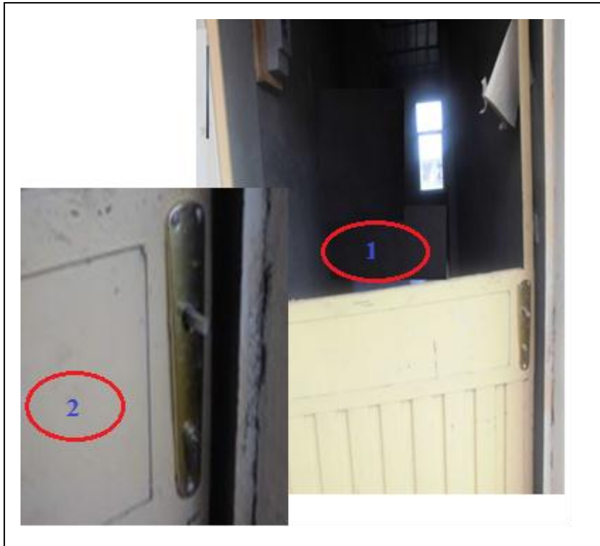
Figure 12: Photographs showing defects on door handle
