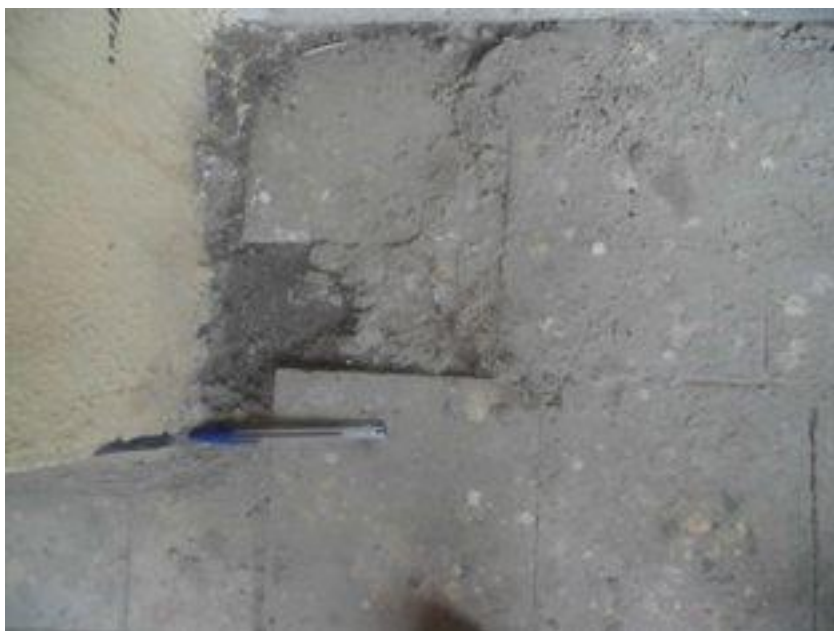
Figure 13: The photographs show tiles delamination of toilet floor
