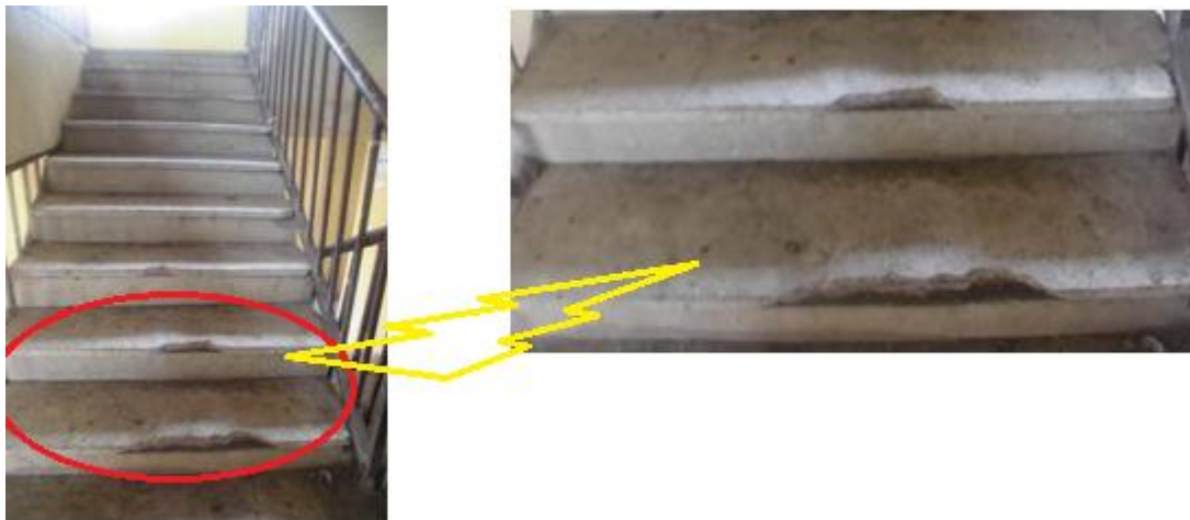
Figure 16: Photographs show defects on the treads of the staircase
