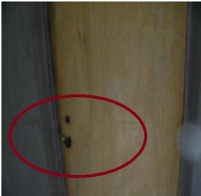
Figure 17: The photo shows a toilet door without the door handle
