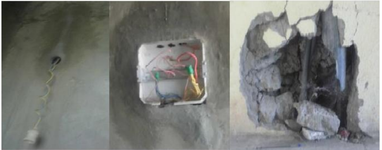
Figure 14: Photographs show defects on electrical fittings.
