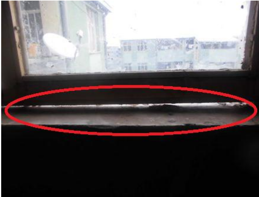
Figure 18: the photograph shows wide opening left between the window frame and the window sill.
