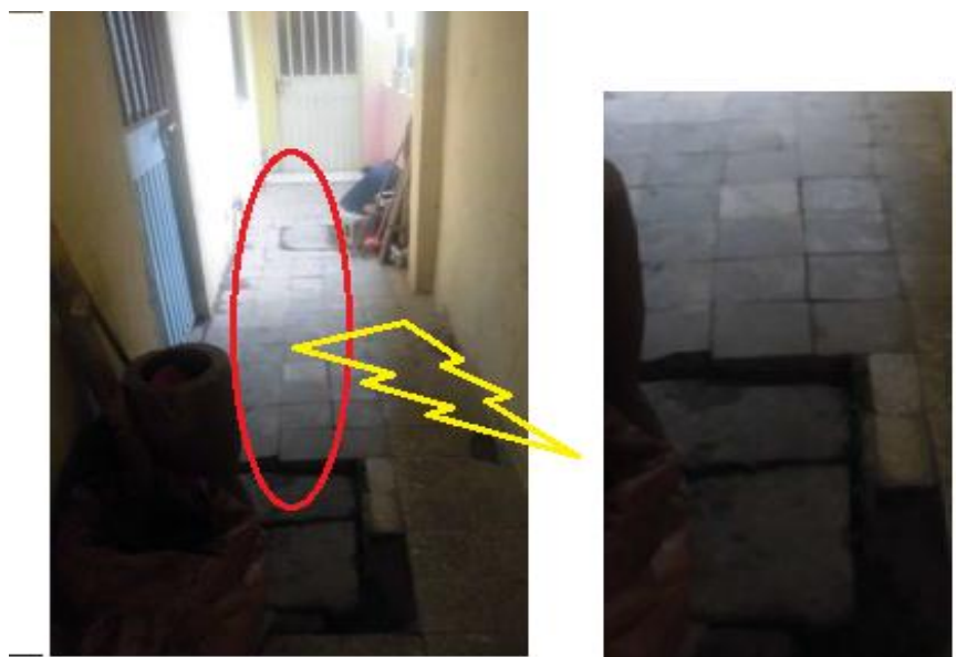
Figure 15: Photographs shows defects on corridor floors
