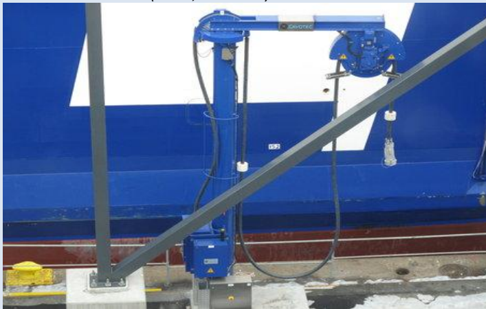
Walstroom in Gothenburg (bron: covatec.com).
