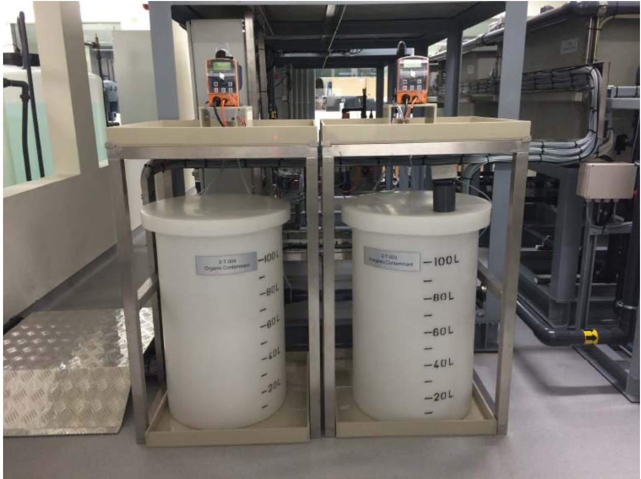
Figure D.7: The contamination tanks with the dosing pumps on top.
