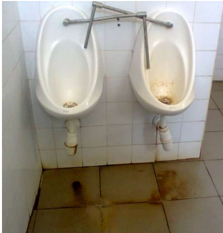
Annex 3 Photograph 5: Plumbing Defects
