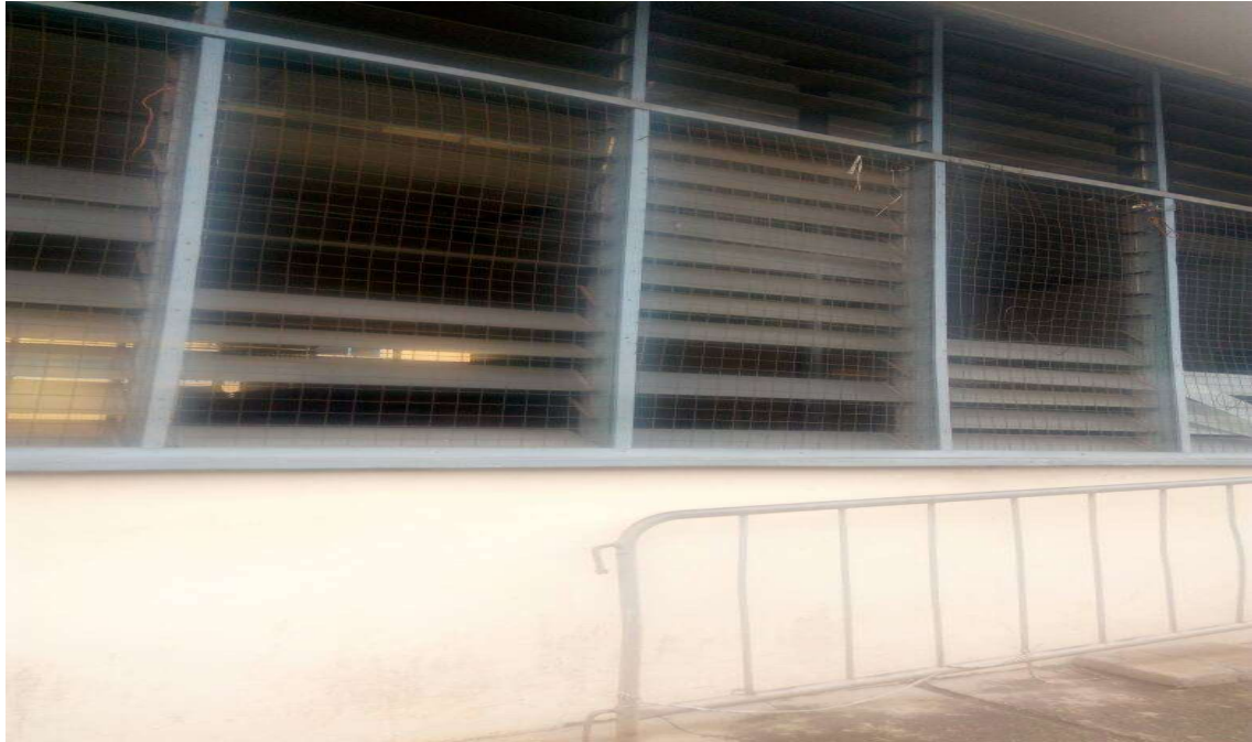
Annex 3 Photograph 2: Window Defects
