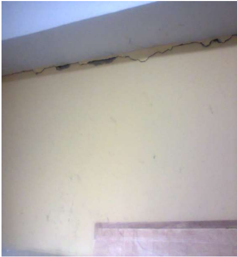
Annex 3 Photograph 4: Cracks in columns and beams
