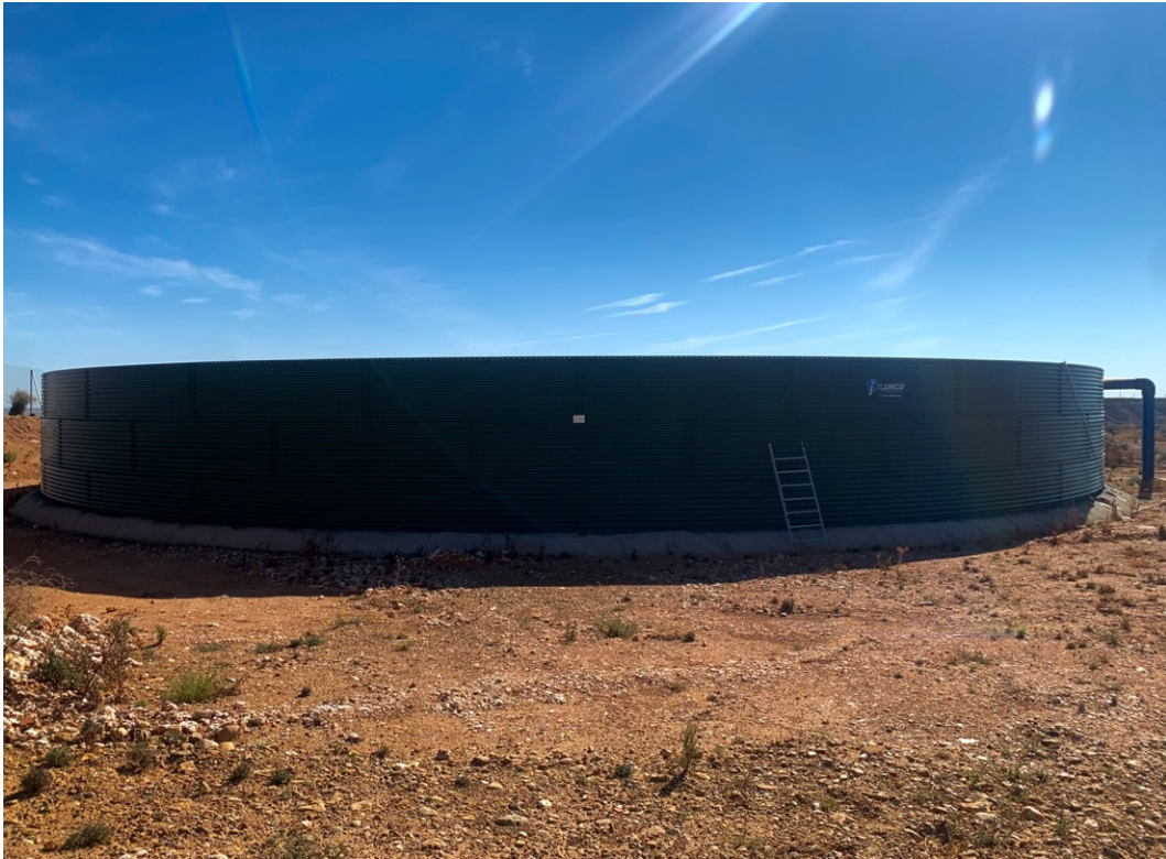
Figure 6 HyPump's reservoir (Source: Fieldwork 2021)
