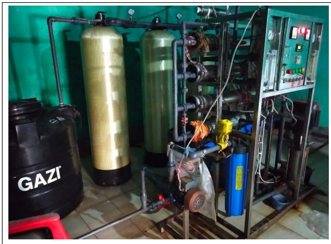
[Figure 7: Desalination Plant]
