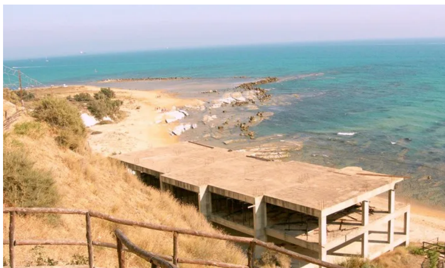
Figure 8: Abandoned and unfinished unauthorised villa in front of beach
