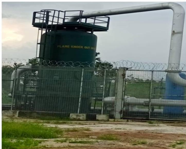
Figure. 4.7: Gas Flaring Facility in Kokori community
