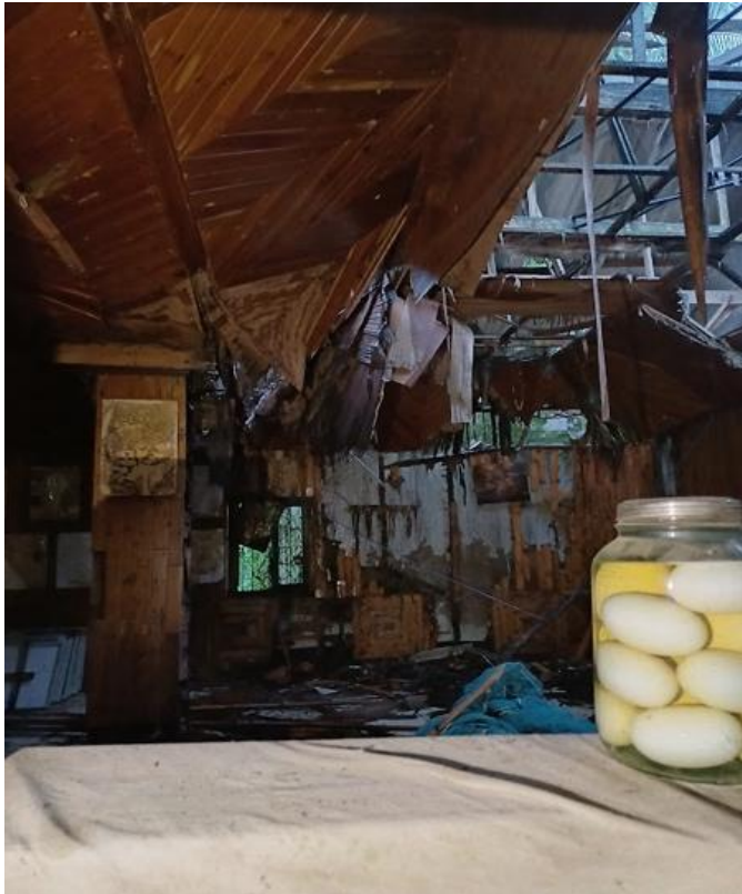
Figure 14. Aftermath of ferocious winds destroys roof of this shelter in this image Source: Photo captured during fieldwork (14 July, 2023)
