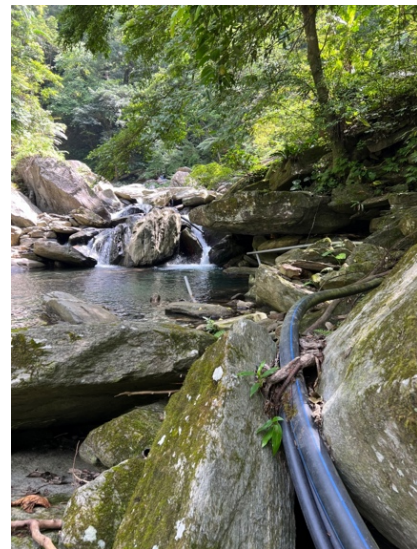
Exposed pipes at AW
