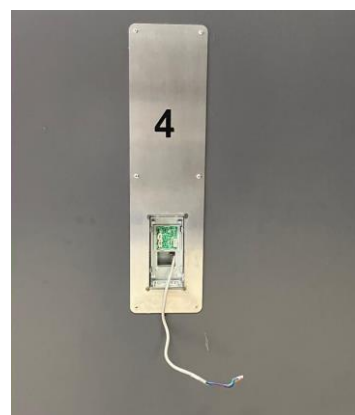
Image 3.1: Missing Elevator Button in Wynberg Courthouse (2023)
