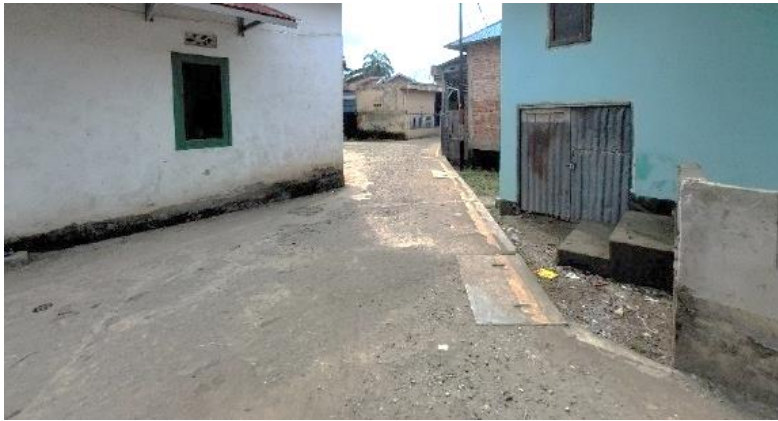
Photograph 15: Road condition after two years
