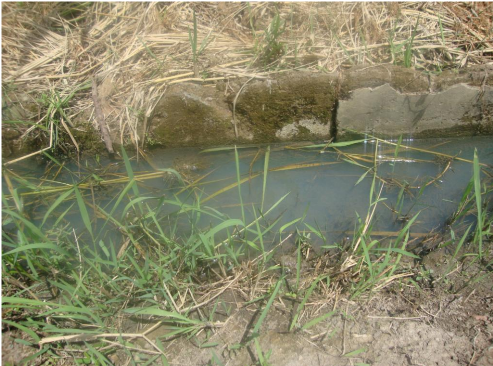
Figure 3.1 A Broken Canal in Karni
