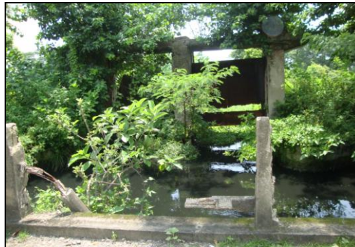
Figure 1.4: The non functional water treatment plant set up earlier at EKW
